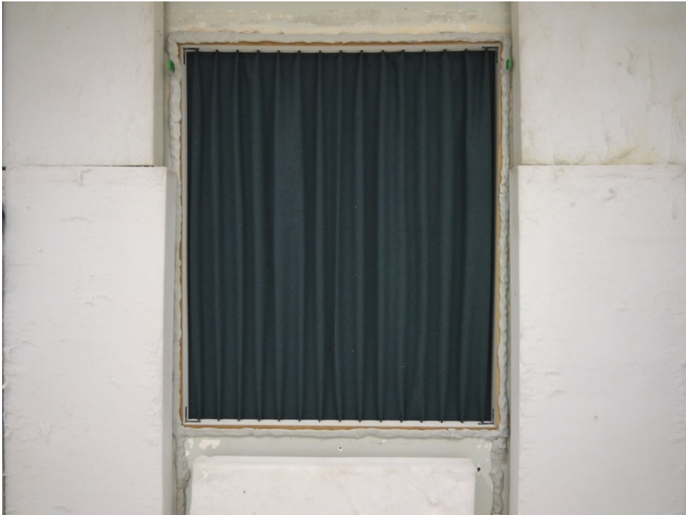
Figure B.1. Exemplary picture of a specimen in the window test stand (reception room side).
